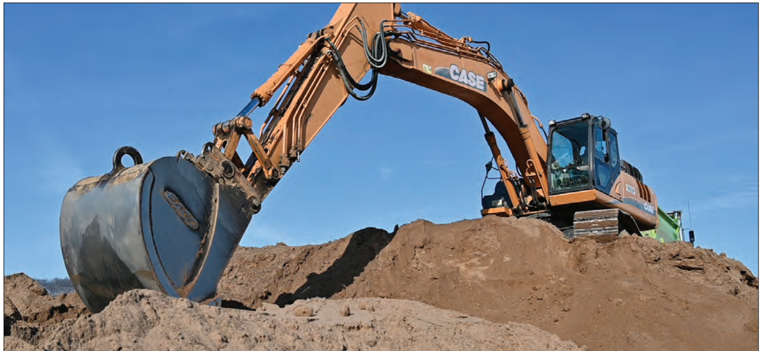
An excavator removes sand from a temporary dredged sand placement site in Wabasha, Minnesota, Jan. 22. USACE St. Paul District photo by Patrick Moes
