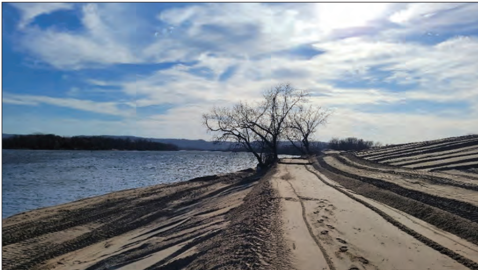
Fisher Island, near Buffalo City, Wisconsin, during construction 2023. USACE St. Paul District photo by Dan DeVaney
