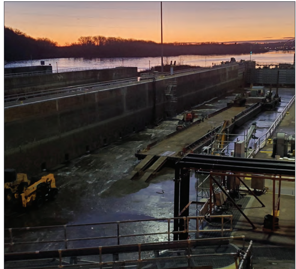
The dewatered lock chamber at Lock and Dam 2 in Hastings, Minnesota, Dec. 13, 2023. USACE St. Paul District photo by Patrick Moes
